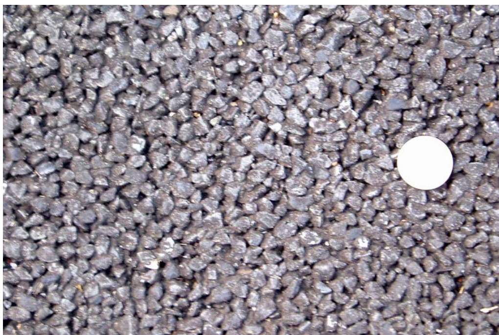
Figure 27. Close up of two layer porous pavement with 8 mm aggregate in the top layer in Yokohama.
