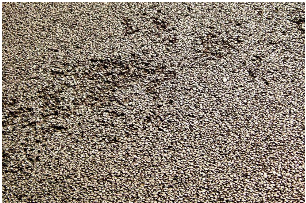
Figure 29. Local areas with ravelling on a new porous pavement in Yokohama.
