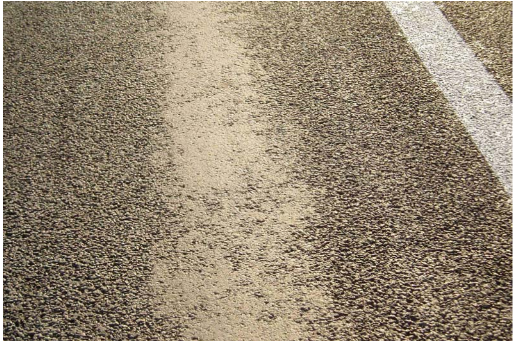
Figure 36. There was a tendency for bleeding of bitumen/mortar in the wheel tracks of the heavy driving lane of the hybrid pavement.
