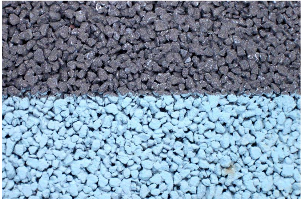
Figure 15. Test sections with porous asphalt. The pavement at the bottom of the picture is painted in a light colour in order to make the pavement reflect the light and heat of the sun in order to reduce the temperature of the pavement in sunny periods. This can prevent rutting of the pavement and reduce temperatures for pedestrians in urban areas.
