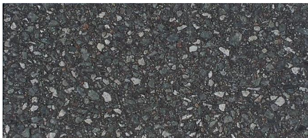
Figure 3: The new road surface on the test site is assumed to be a dense graded asphalt concrete with soft binder
